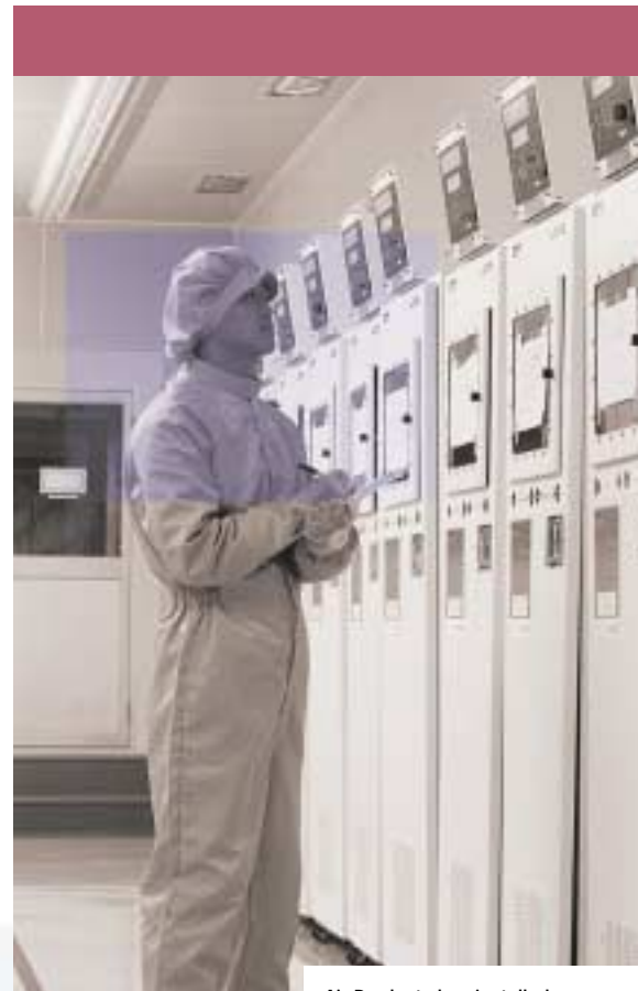
Air Products has installed more than 6,000 GASGUARD systems around the world for more than 100 semiconductor manufacturers.
