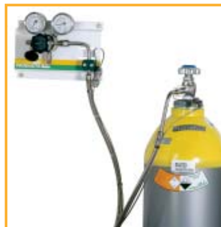
Gas cylinder connected to a regulator mounted on panel
