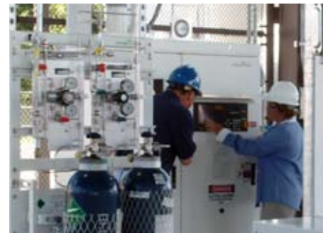
Air Products’ technicians monitors the performance of a BSGS system for White Amonia.
