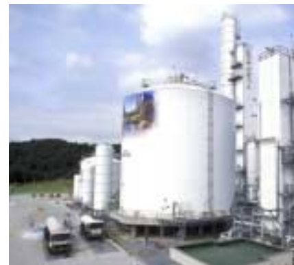
Air Products will build two more air separation units (ASUs) like this one at Tangjung, Korea to serve Samsung's expanding needs.
