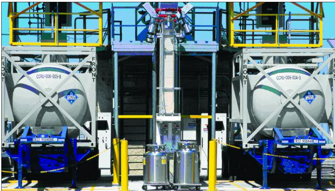
Figure 1: BSGS Installation of Bulk ISO Supply
