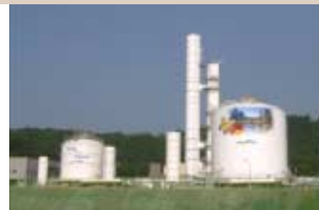
Air Products' air separation plant at Samsung's new facility in Tangjung will supply five to eight times the amount of Nitrogen that a typical semiconductor fab consumes.
