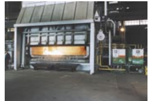
Figure 7: Looking into the charging chamber of an APMELT TCM™ twin-hearth furnace
