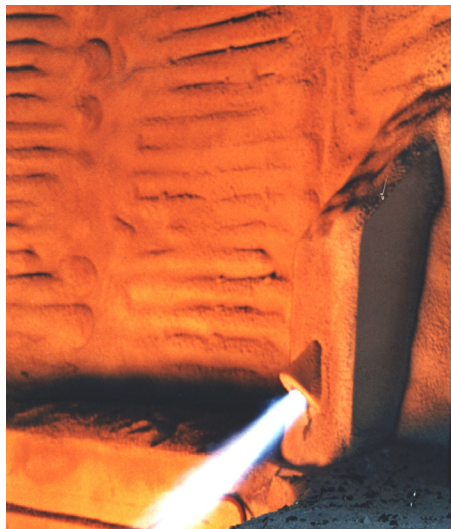
Figure 2: Key to the success of the JetBOx™ technology is the combination of a shrouded oxygen jet with a special mounting that places the jet nozzle much closer to the metal surface. Because the oxygen jet has to travel a shorter distance, it is still supersonic when it strikes the surface of the molten metal. Penetration is greatly improved, giving faster decarburisation and more efficient use of oxygen
