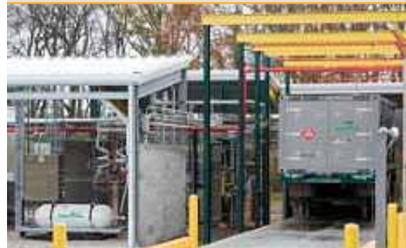
Air Products’ Silane transfill facility in Hometown, Pennsylvania.
