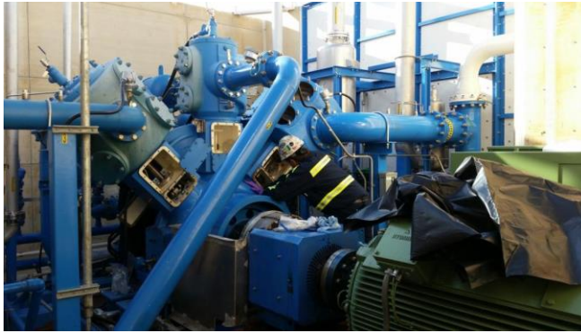
Reciprocating Compressor Maintenance – Virginia, USA
