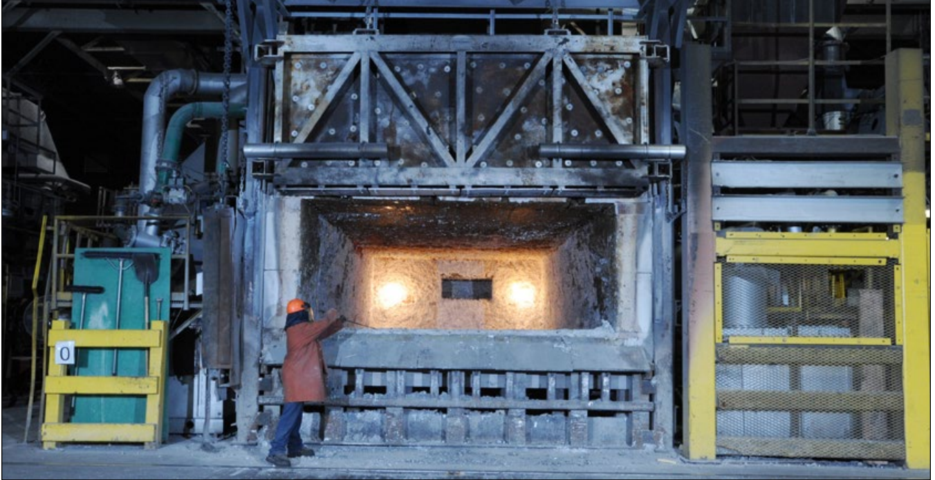
Reverberatory furnace at Sapa fitted with adjustable heat release oxy-fuel burners.
