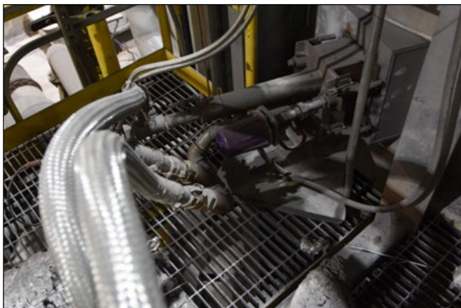
Figure 5. Adjustable heat release oxy-fuel burner installed in Sapa's 65,000 lb reverberatory furnace.
